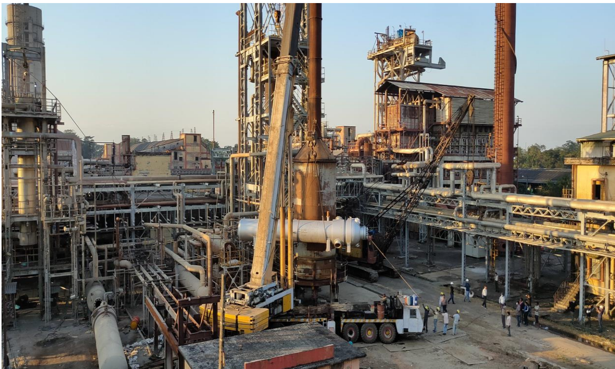
Replacement of the old Water Cooled Condenser with a new one in Annual Shutdown 2020
