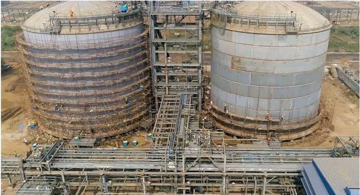
HURL-Barauni- Ammonia Storage Tank
